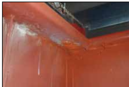
Original coating started to fail within 12 months of application.
