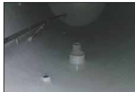
Coated tank internals.
