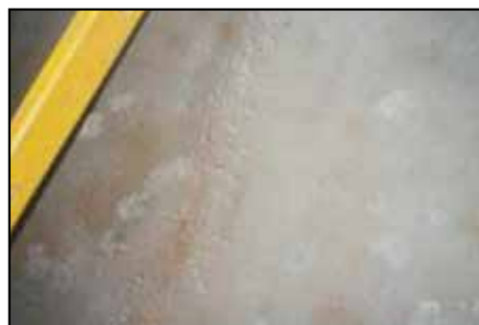
Corrosion and pitting on the spillway gate.
