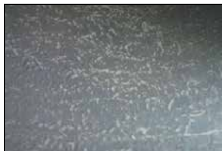
Corroded tank internal surface.
