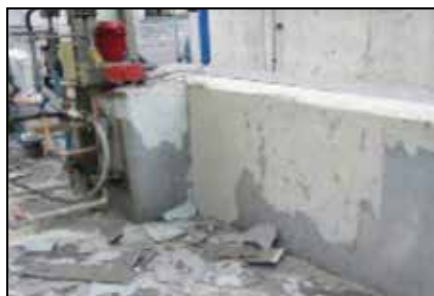
Failed coating after spills.
