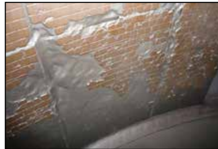
Damaged pulverizer walls.
