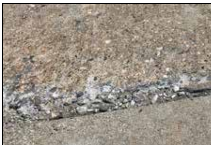
Damaged concrete surface.
