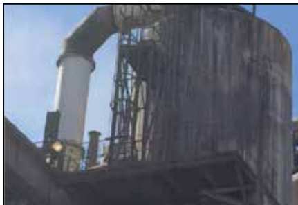
Flash cooler with exhauster.
