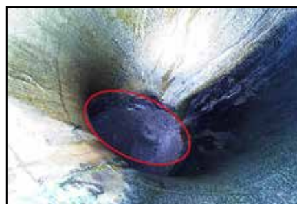
Dark scale formation on unlined section.
