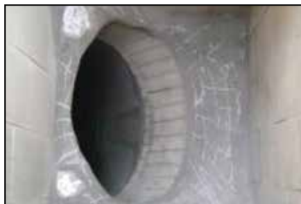
Damage to existing ceramic tiles caused unscheduled shutdown and loss of production.
