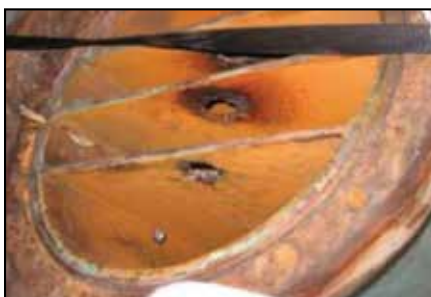
Corroded divider plates.
