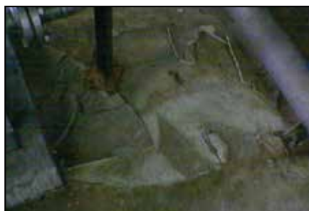
Delaminated fiberglass mat polyester.
