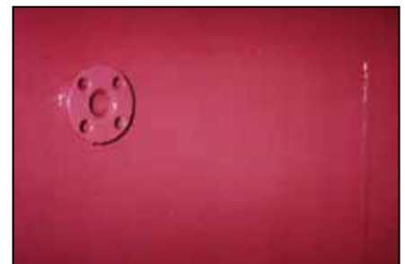
After proper surface preparation, ARC S4+ was applied in a two-coat system.
