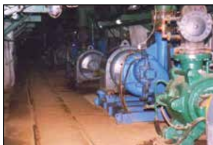
Bank of dewatering pumps.
