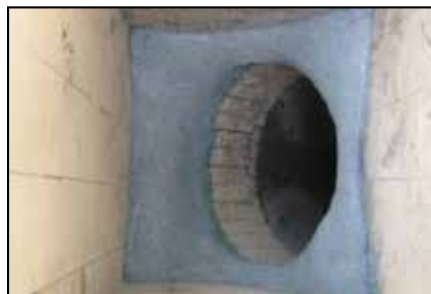
Installation of ARC BX5.
