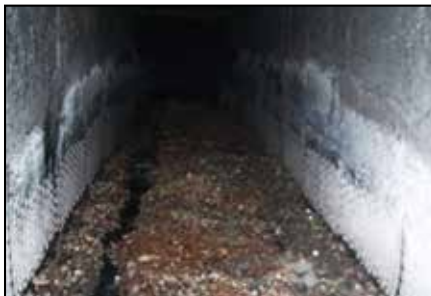
Discharge flume with damaged tile/rubber liners.
