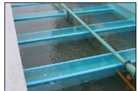
Sand filter in service.
